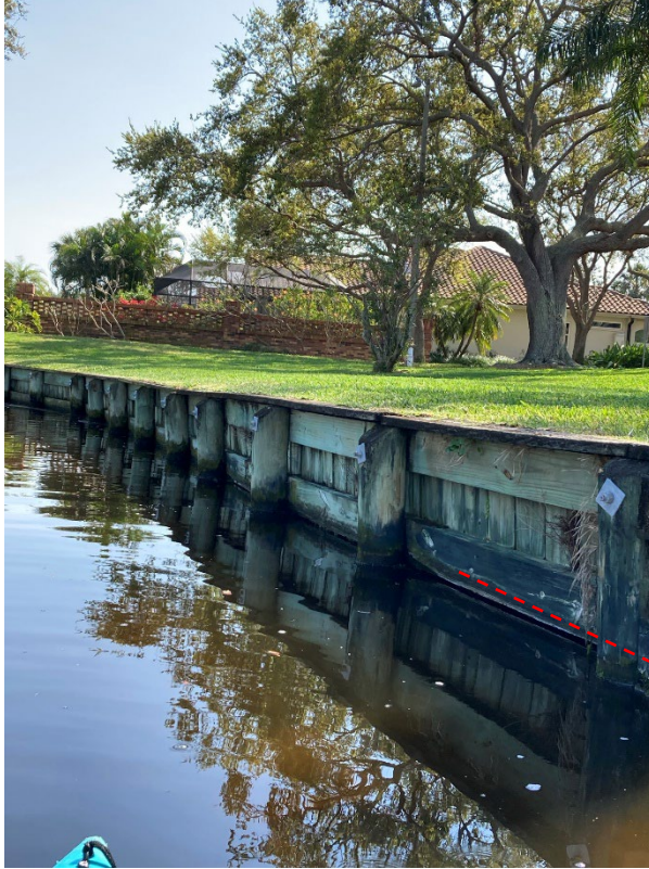
Photo 7: View of Bowing Walers and Leaning Wall in Pond #9
