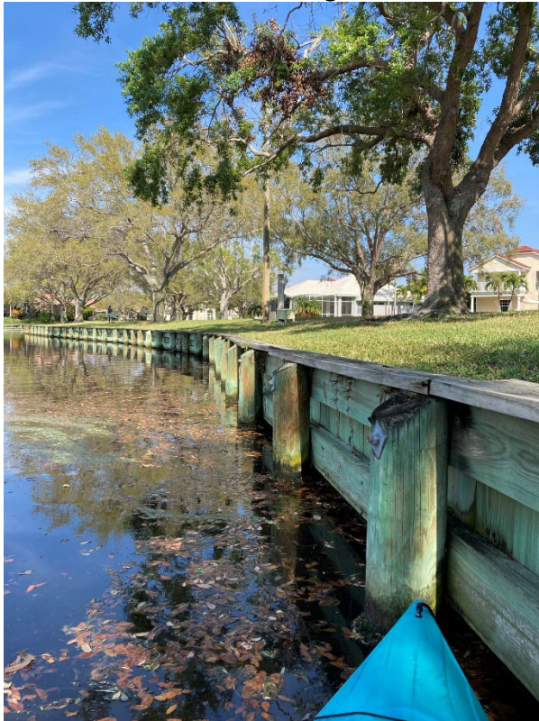
Photo 8: View of Bowing Walers and Leaning Wall in Pond #9
